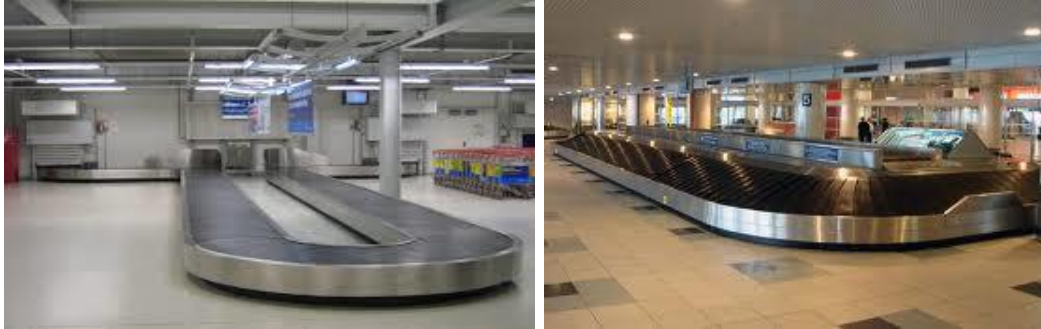
FIGURE 31: Baggage claim conveyor, horizontal plates (a) and central supply and sloped plates (b)
