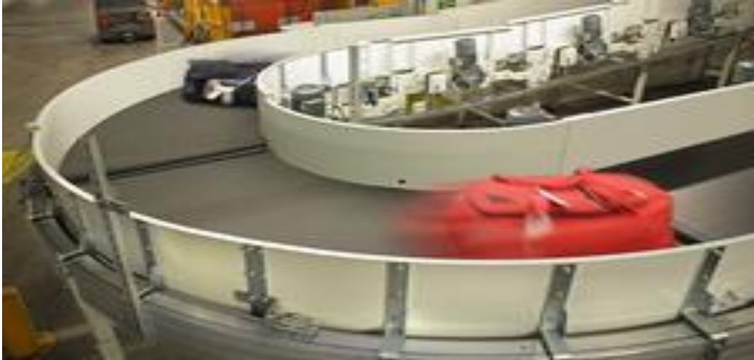
FIGURE 16: Belt curve conveyor system
