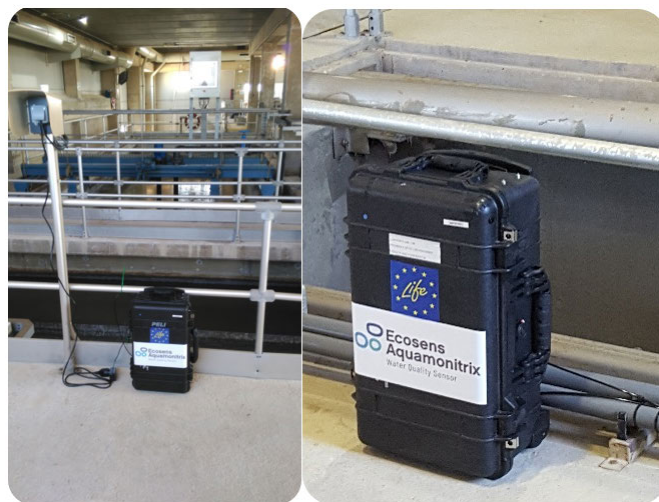
Fig. 1. Pictures of the IoT device deployed at WWTPs.
